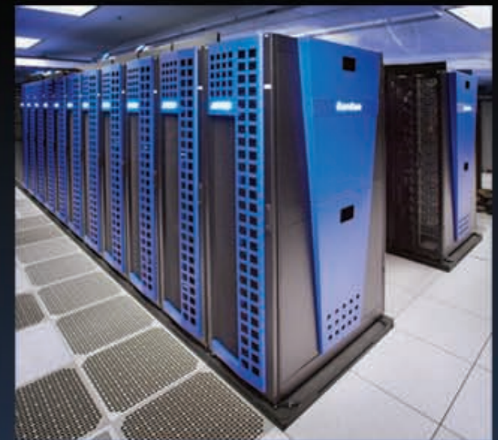
SDSC'S GORDON SUPERCOMPUTER. PHOTO: ALAN DECKER.
