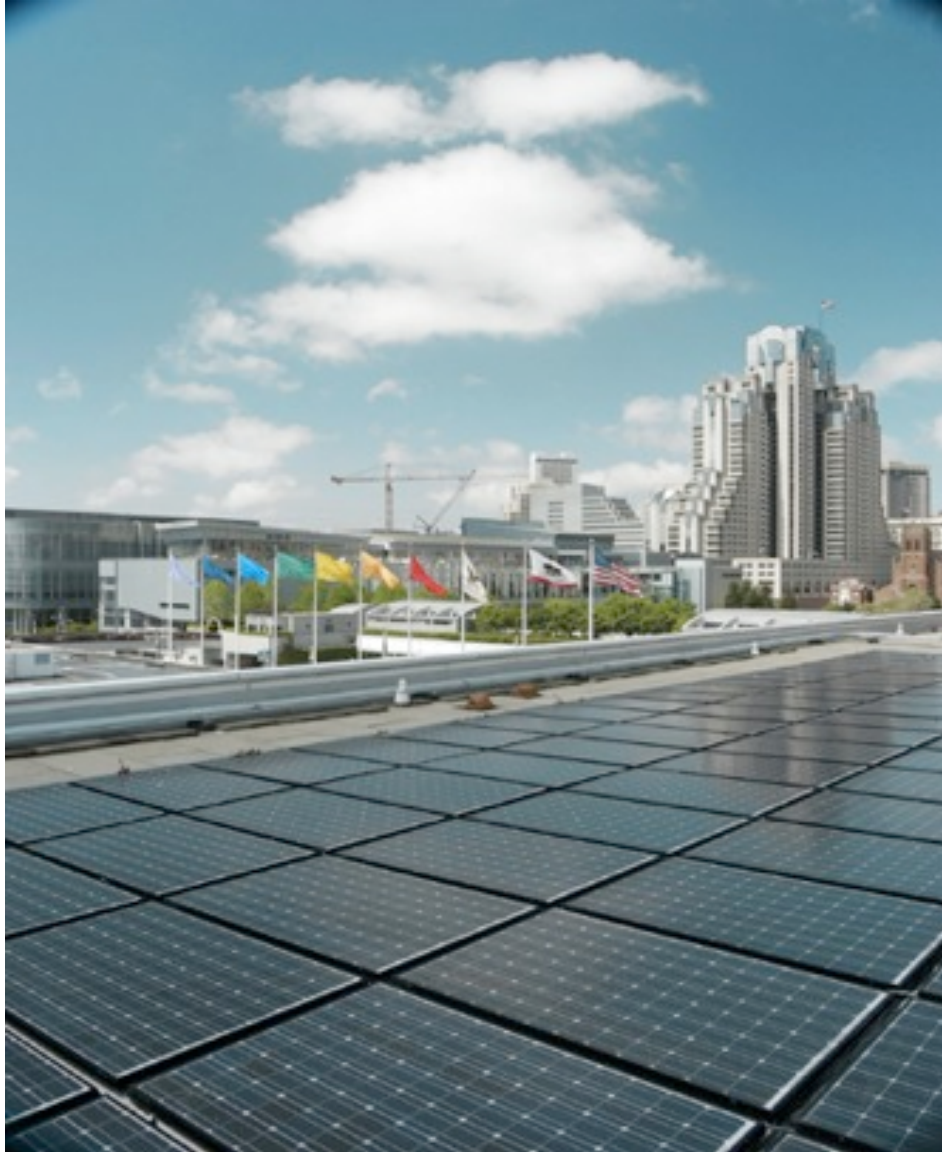
Moscone Center's Solar roof panels
